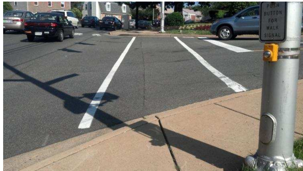
Crosswalk without curb ramp (both sides)
