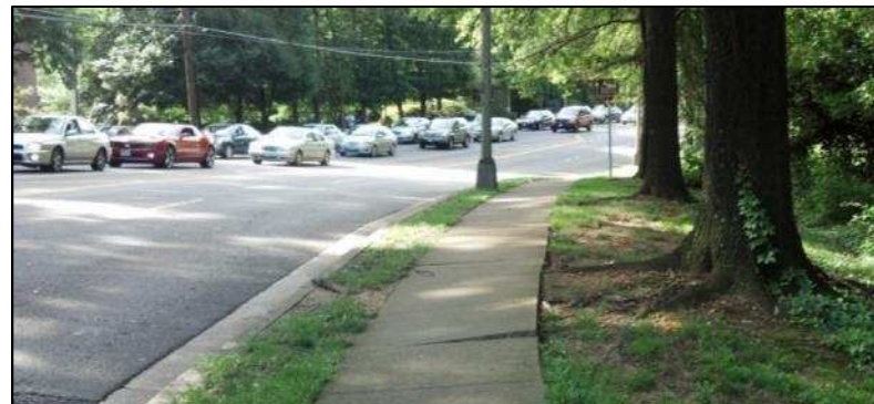
Tree roots causing sidewalk unevenness along Carlin Springs Rd
