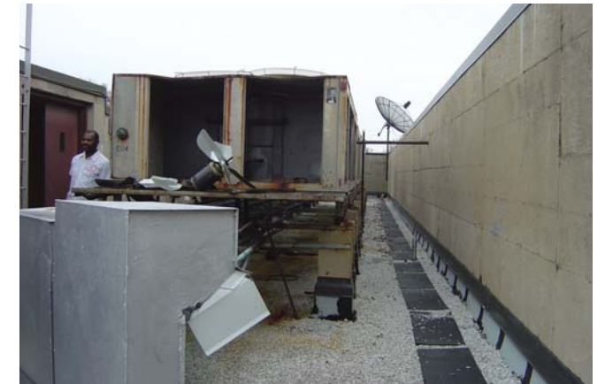
Roof Top Mechanical Equipment
