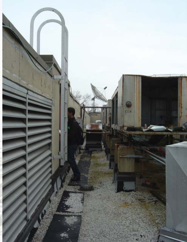
Roof Top Mechanical Equipment
