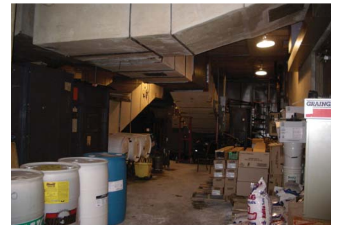
Mechanical Room - Interior
