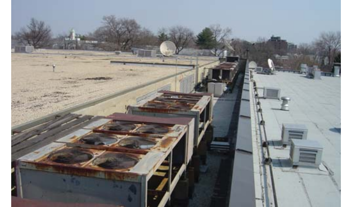
Roof Top Mechanical Equipment
