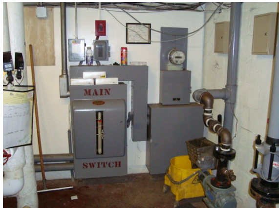
Photo #24: Electrical switchgear
