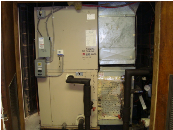
Photo #21: Air handler
