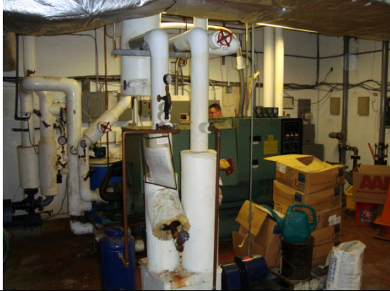
Photo #19: Mechanical room
