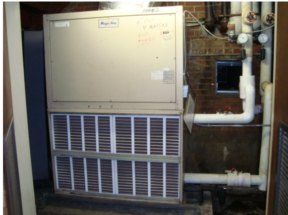
Photo #22: Air handler
