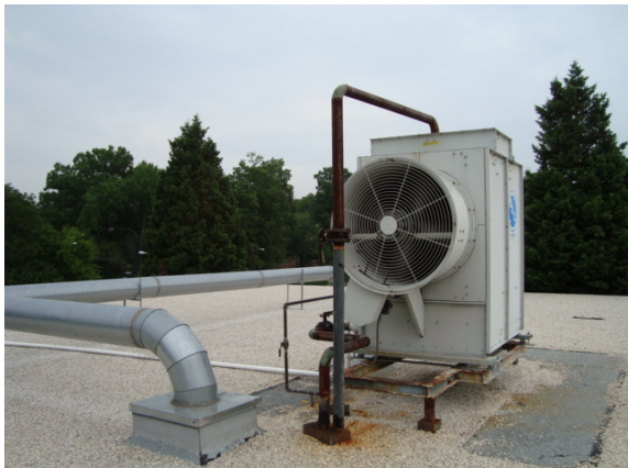
Photo #17: Cooling tower
