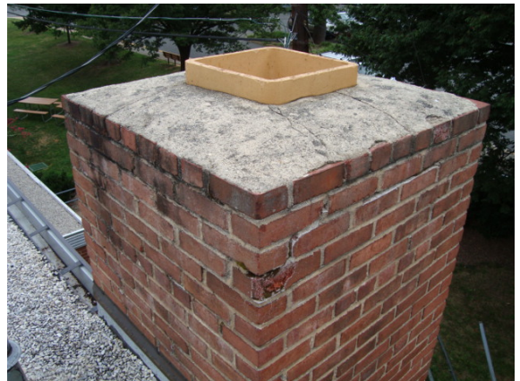
Photo #18: Chimney - note deteriorated masonry
