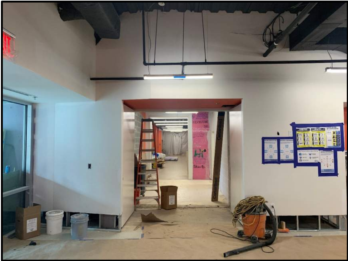
View of new connection between new and existing parts of the school
