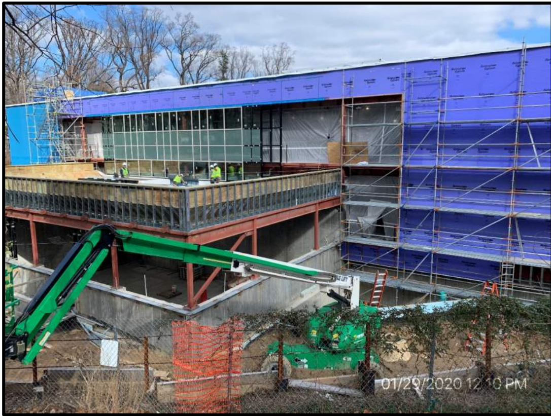
West elevation of building with curtain wall, auxiliary gym, and site works
