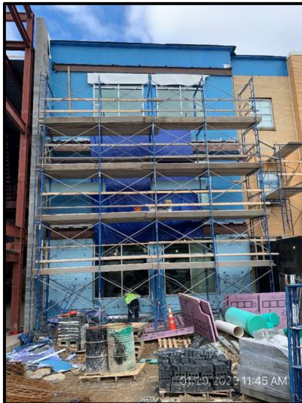
South elevation of renovation façade where new gray brick façade is to be installed
