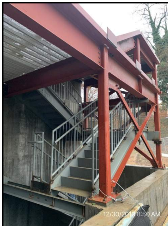
Current status of stair "1" at rear of auxiliary gym.
