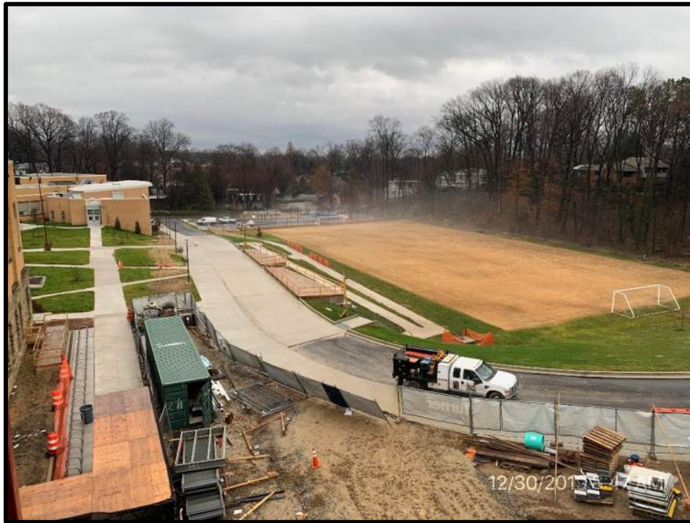
Current state of landscaping and athletic field at the rear of the school. Note bicycle racks in the bottom left of the photo which are used by students.
