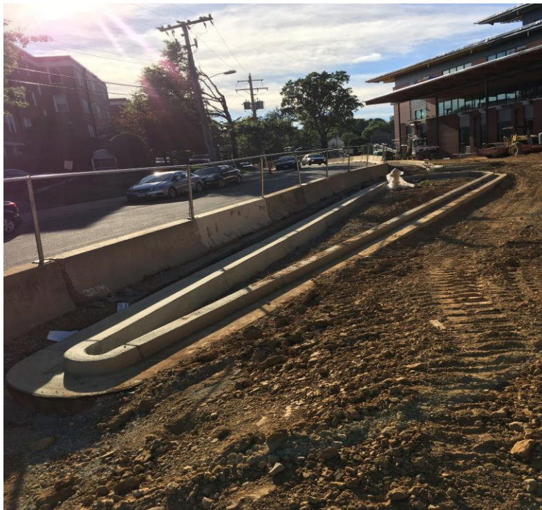
NEW CURB AND GUTTER FOR DROPOFF/PICKUP LOOP OFF OF S OLD GLEBE RD
