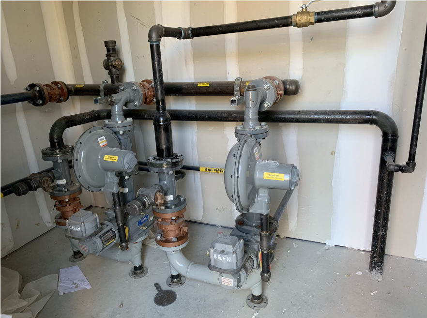
Gas meters installed
