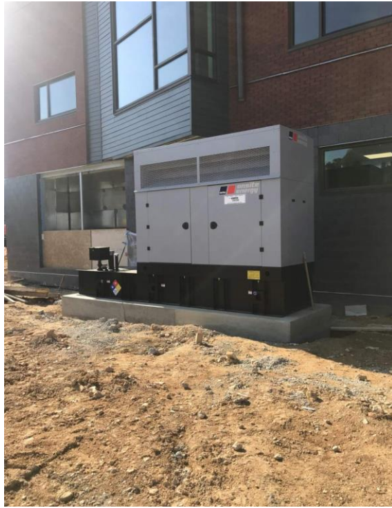
EMERGENCY GENERATOR SET
