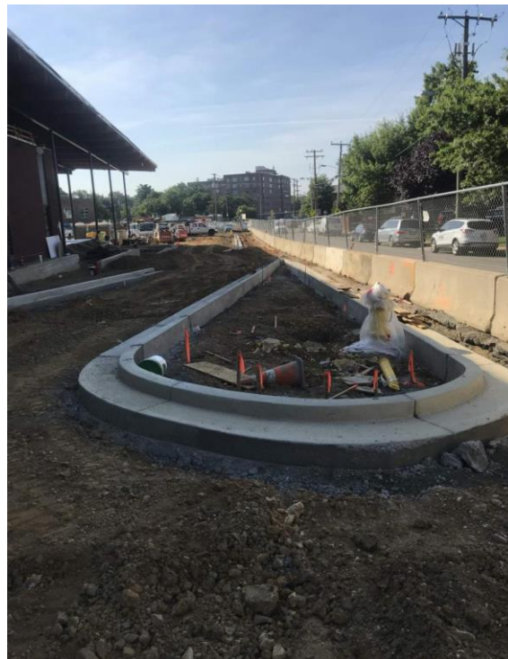
NEW CURB AND GUTTER FOR DROPOFF/PICKUP LOOP OFF OF S OLD GLEBE RD
