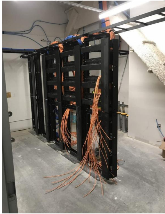
SECONDARY COMMUNICATIONS ROOM
