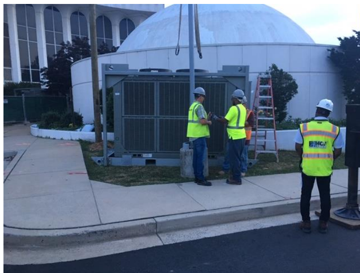
Planetarium Temporary Chiller Set Up
