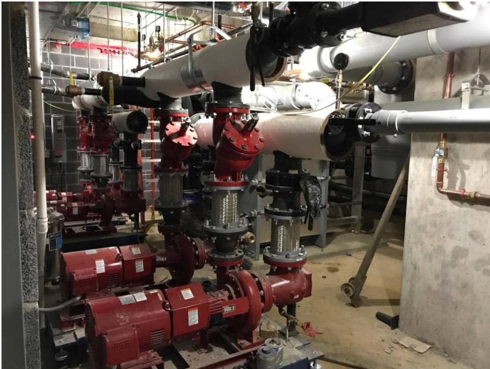
GEOHERMAL PUMP ROOM ON UPPER LEVEL OF GARAGE
