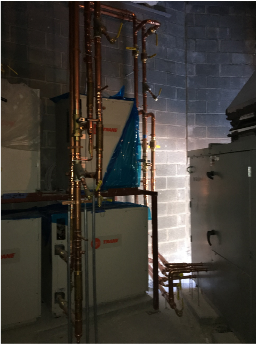
Mechanical equipment installed at level 5
