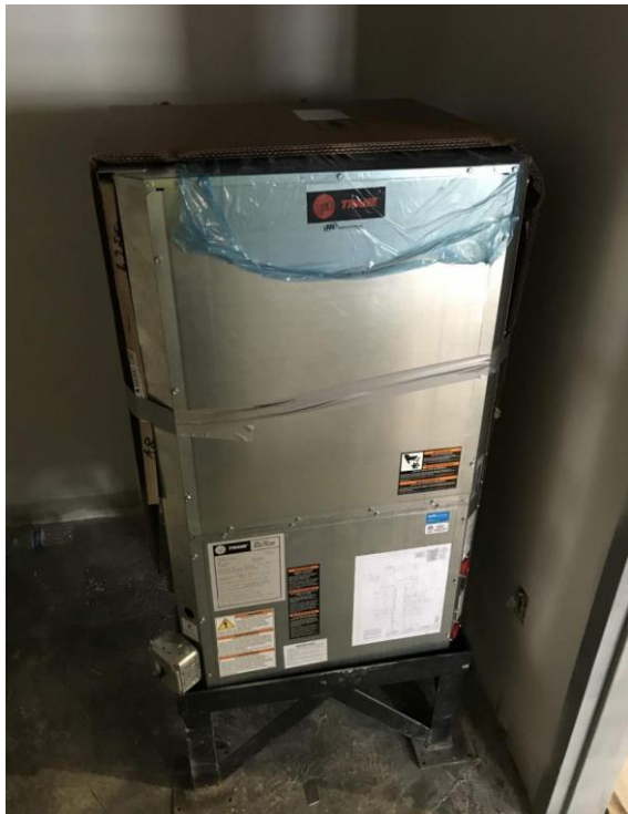
SETTING OF INDIVIDUAL CLASSROOM WATER SOURCE HEAT PUMPS
