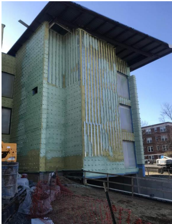
INSTALLED FAÇADE CLADDING NAILERS ON TOP OF SPRAY FOAM/AIR BARRIER AT FAÇADE ABOVE GARAGE ENTRY
