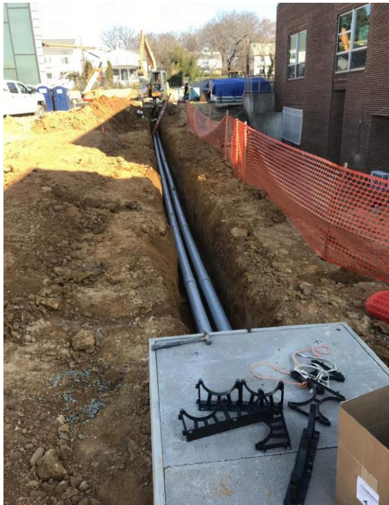
PRIMARY ELECTRICAL SERVICE CONDUIT AND PULL BOX
