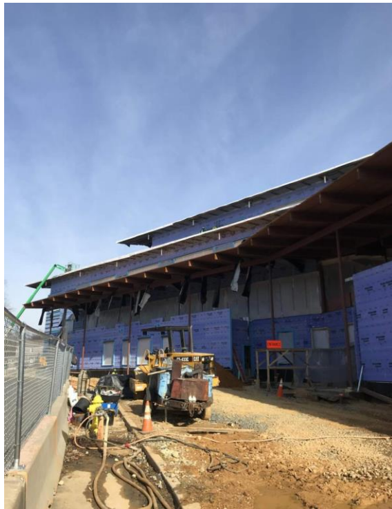
COMPLETION OF STRUCTURAL WOOD ROOF AND CONSTRUCTION OF EXTERIOR WALLS AT FAÇADE ADJACENT TO S OLD GLEBE RD
