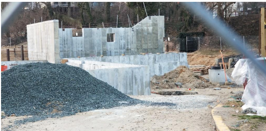
North Elevation of Addition (looking at exit stairway / gym storage room at Auxiliary gym)
