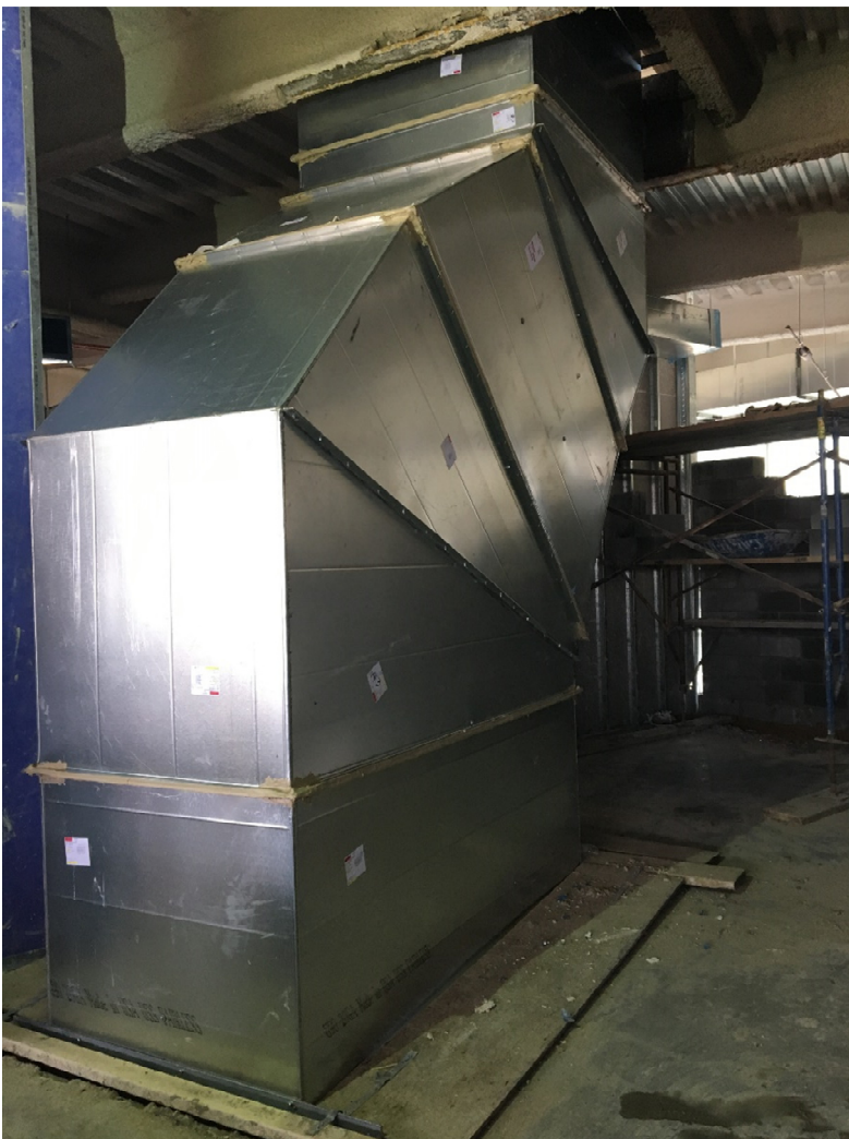
Smoke exhaust duct at L4
