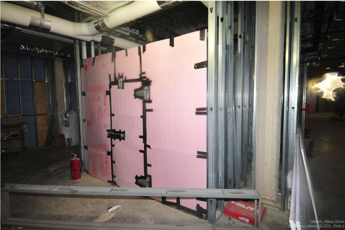
Walk in and freezer and cooler installed
