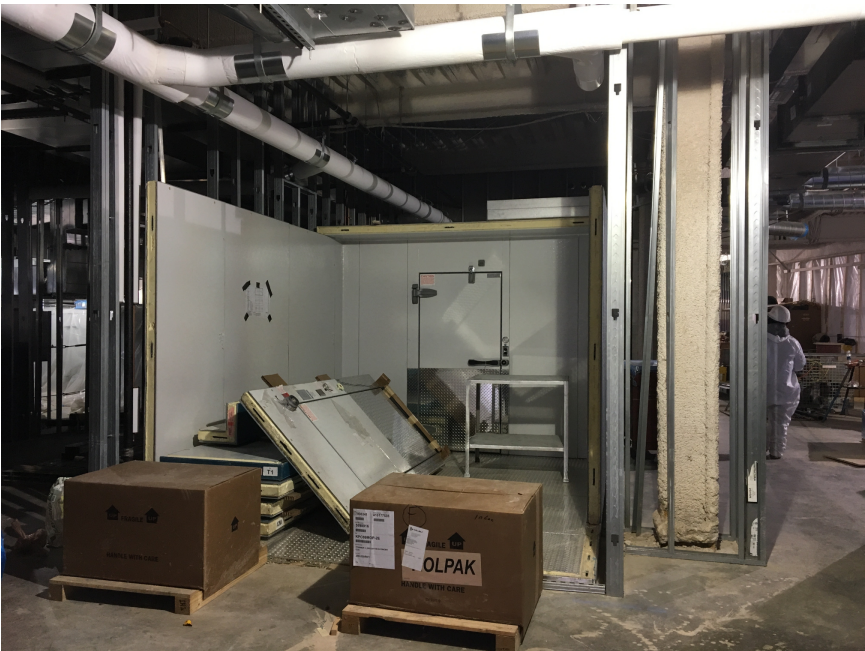
Walk-in cooler and freezer installation
