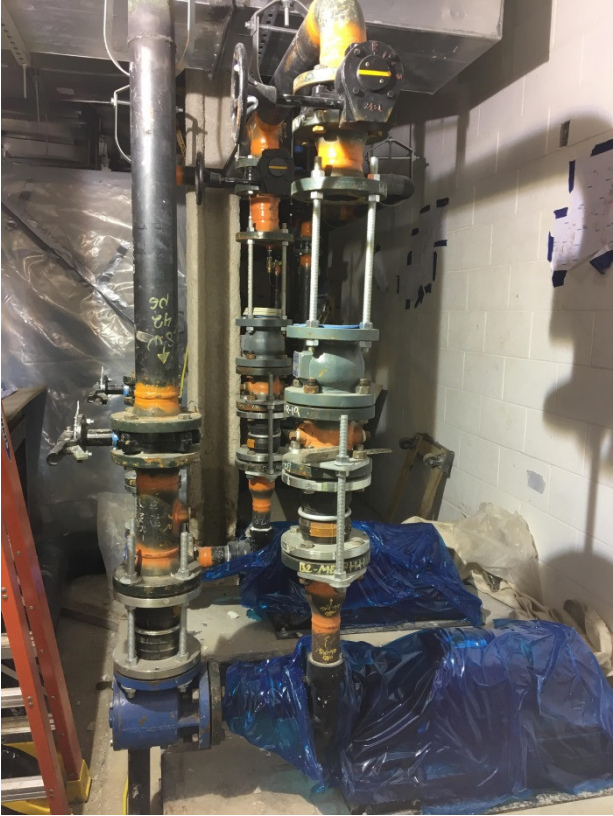
Mechanical room pipes
