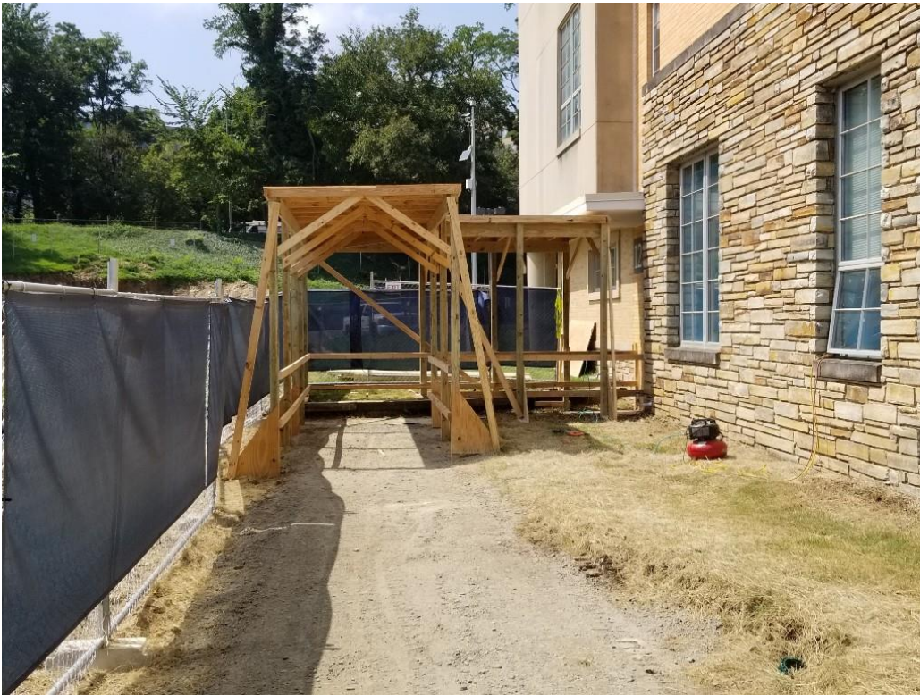
Temporary emergency egress canopy from Door 12
