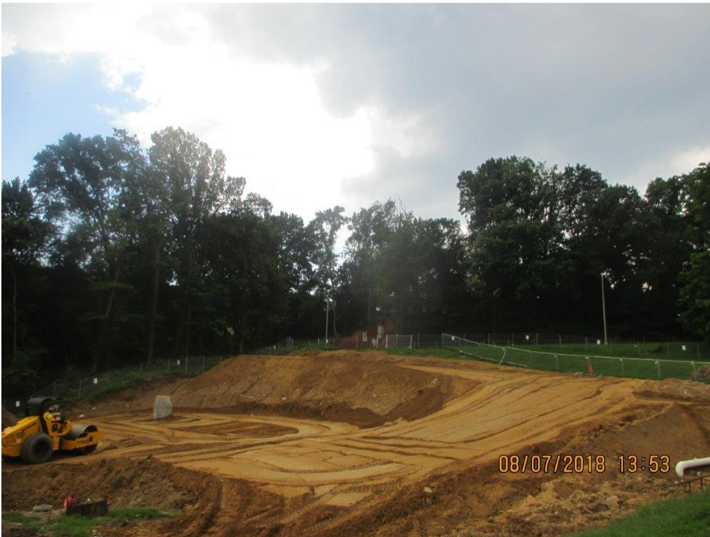
View from school towards Old Dominion Drive looking at future Drop Off Road
