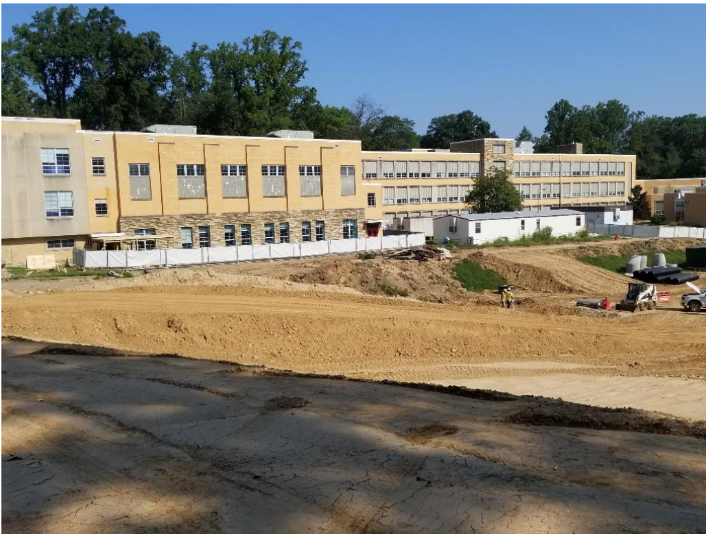
View from Old Dominion Drive atop future Drop Off Road towards school
