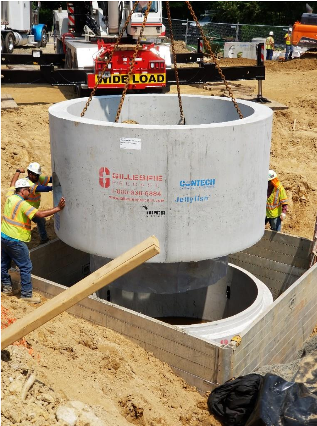
Future underground "Jellyfish" Storm water filtration system
