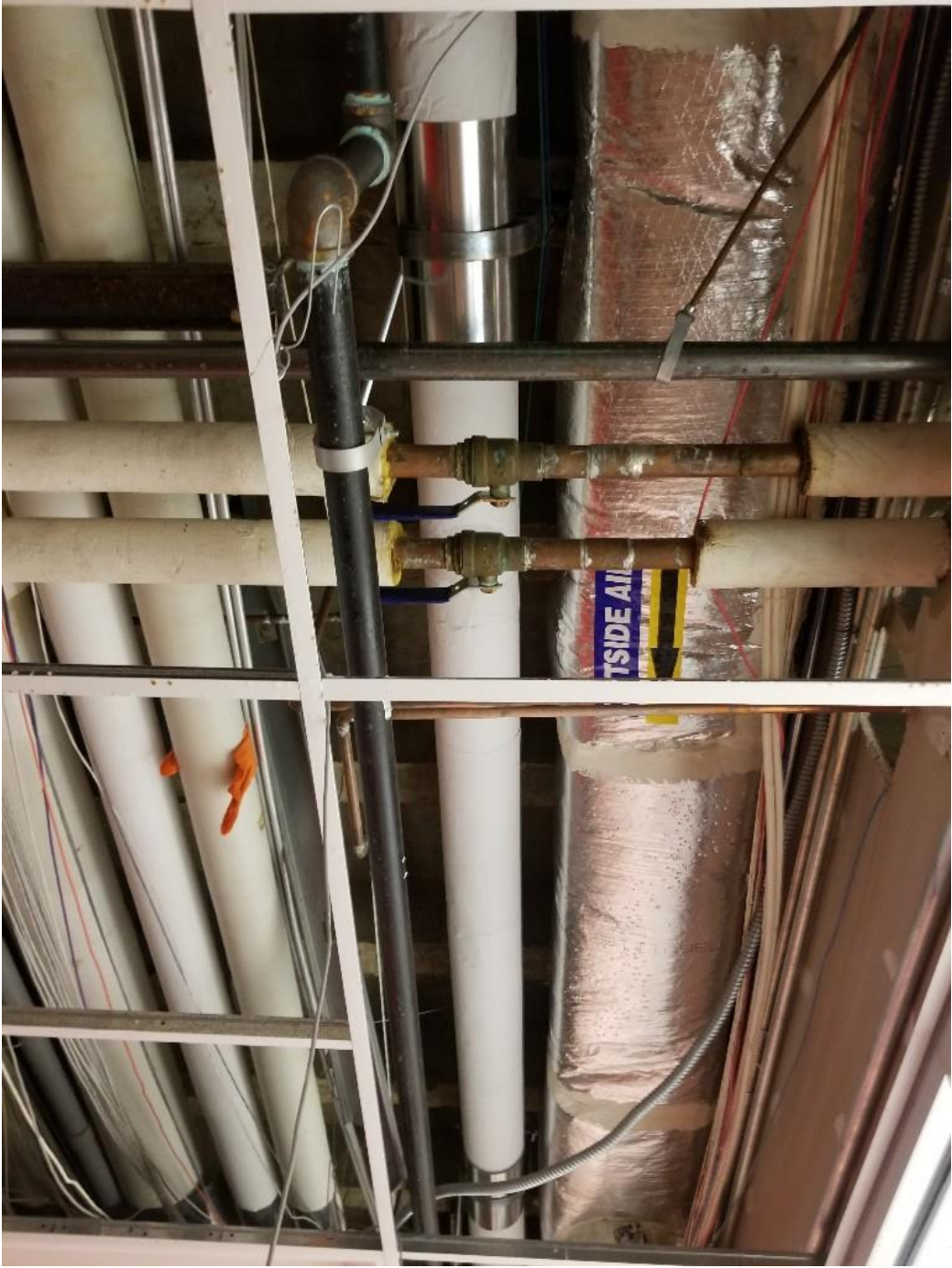
Portion of new electrical and mechanical piping system from Existing building stubbed-out to new addition
