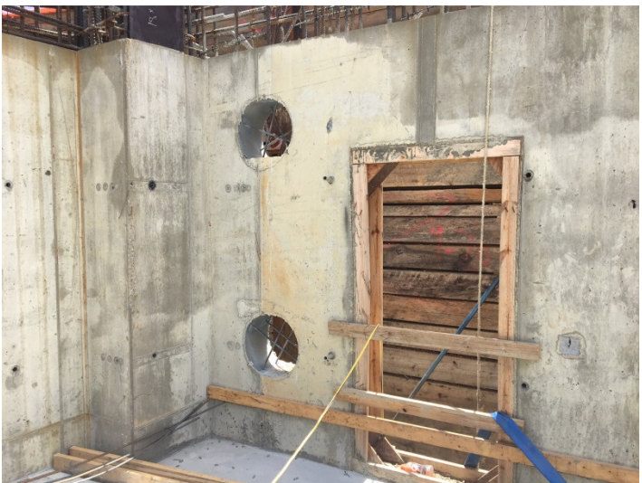
Sleeves and entrance to DVP vault
