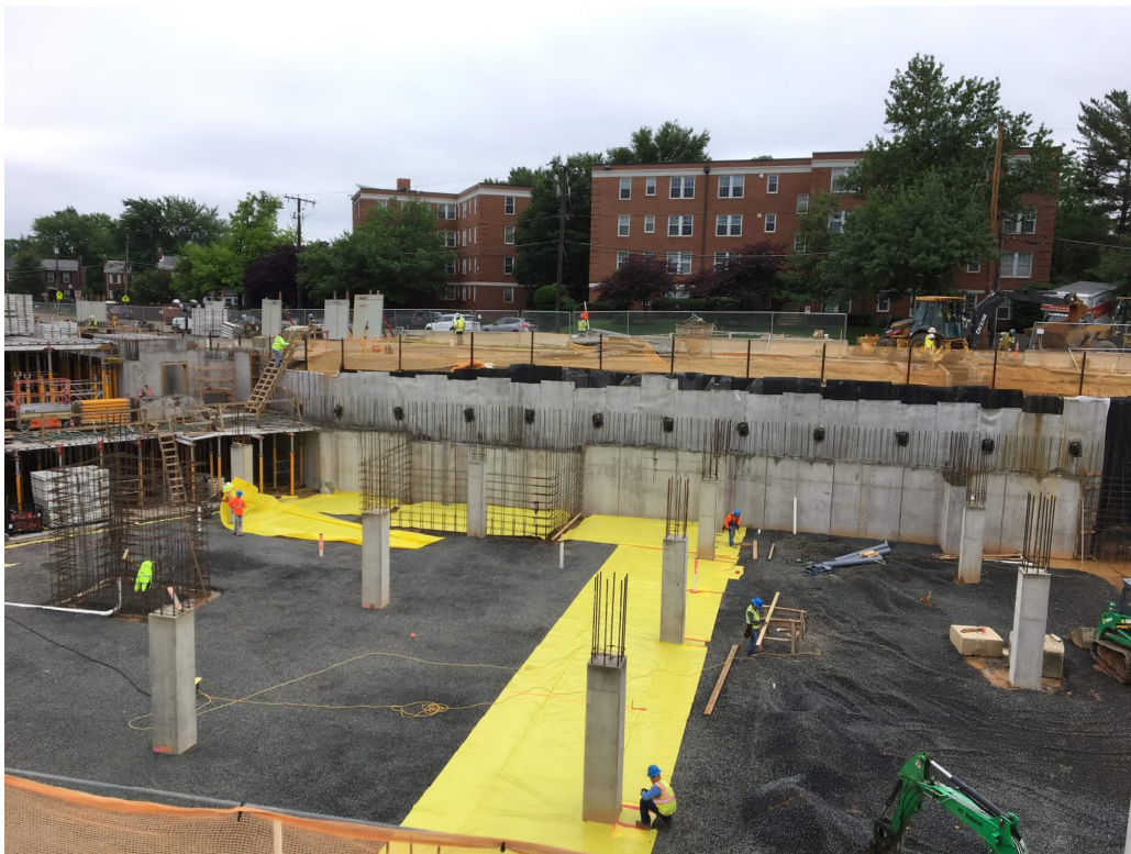
PREP OF STONE BASE AND VAPOR BARRIER UNDER GARAGE LOWER LEVEL SLAB
