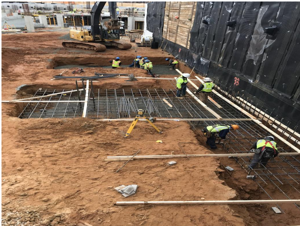
ONGOING WATERPROOFING OF GARAGE WALLS AND INSTALLATION OF REINFORCING STEEL AT GARAGE LOWER LEVEL FOOTING
