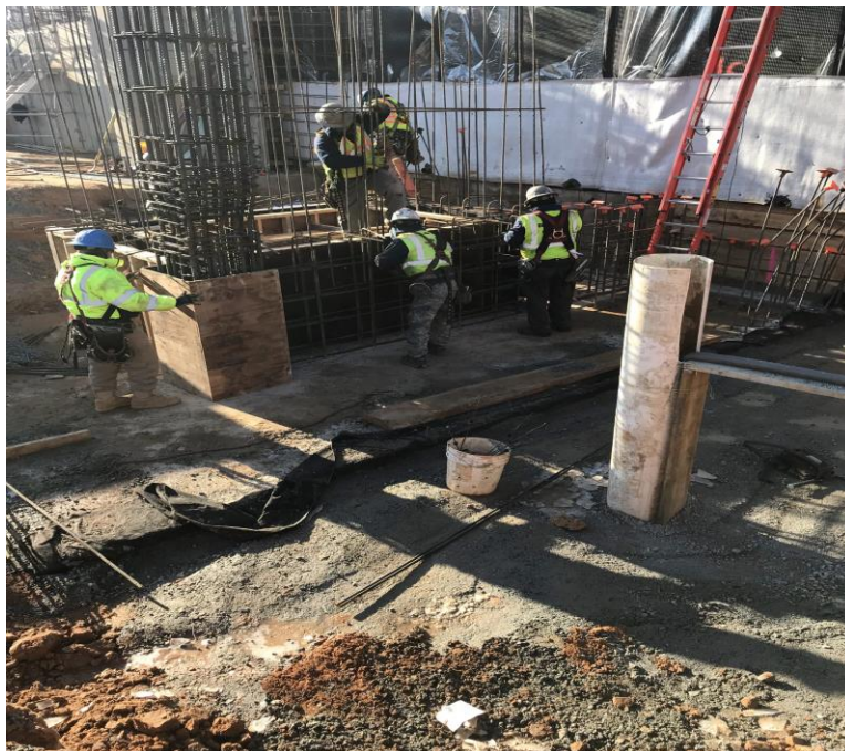
INSTALLATION OF REBAR AT FOUNDATION WALLS AND COLUMNS PRIOR TO PLACEMENT OF FORMWORK
