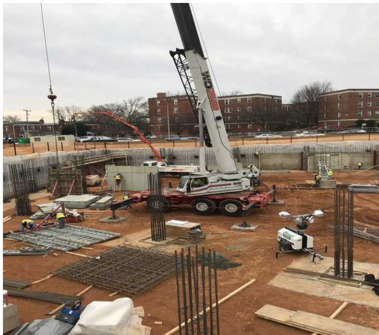
MOBILE CRANE MOVING MATERIALS FOR INSTALLATION OF FOOTINGS AND FOUNDATIONS AT LOWER GARAGE LEVEL
