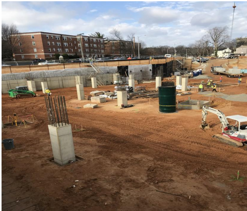
PREPPING FOR PLACEMENT OF PRE-FABRICATED SUMP PIT STRUCTURE AT LOWER LEVEL OF GARAGE
