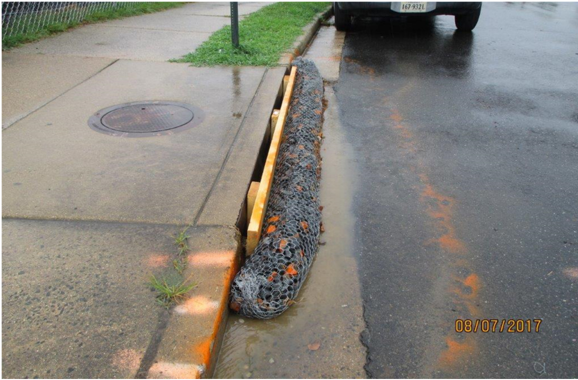
EROSION AND SEDIMENT CONTROLS INLET PROTECTION
