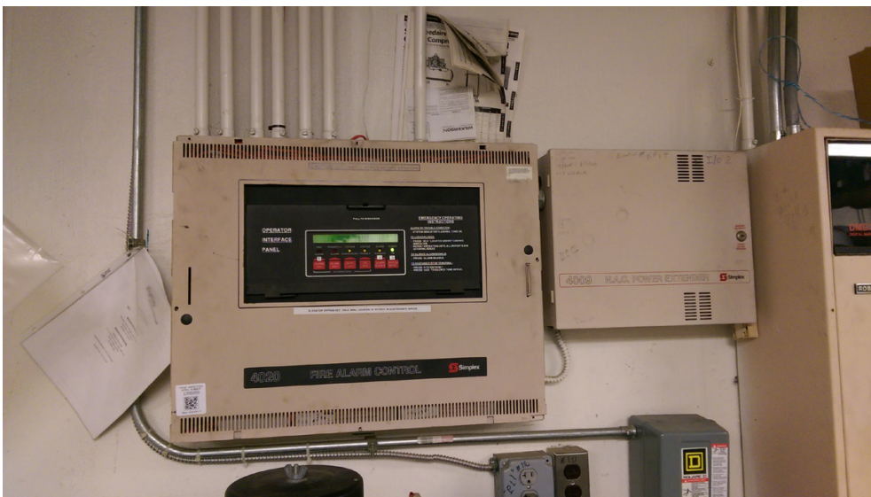
Existing fire alarm control panel and equipment
