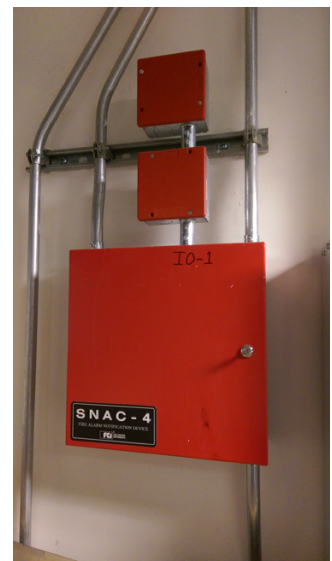
Typical fire alarm NAC panel
