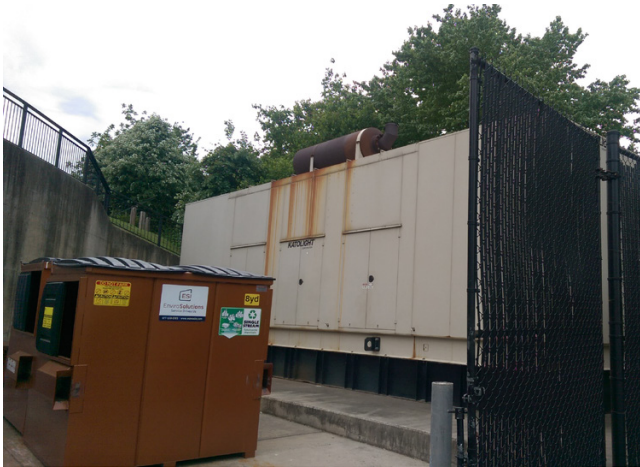
Existing generator and fenced enclosure
