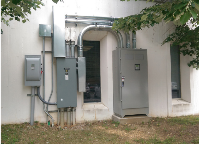
Existing electrical main disconnect along exterior north wall
