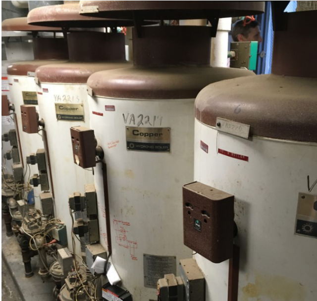
Gas fired boilers
