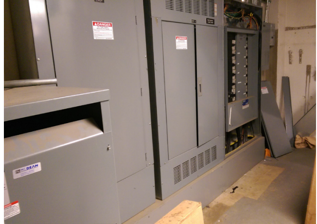
Existing electrical main switchgear in mechanical room
