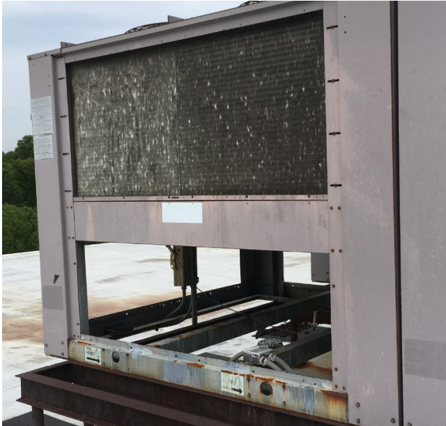
Outdoor condensing unit
